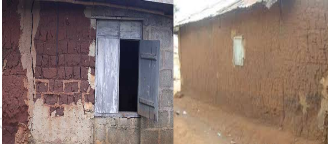
Figure 2.9: Wall of a Traditional Building that Cracked after Frequent Years of Rain-fall
